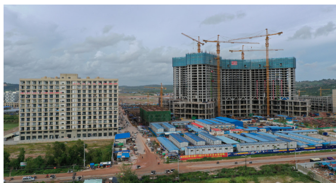
Chinese buildings and condominiums are being constructed on several hectares of land along the Otres Beach in Sihanouk province
